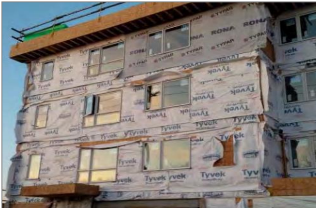
Figure 2.5 Poor House Wrap Installation
